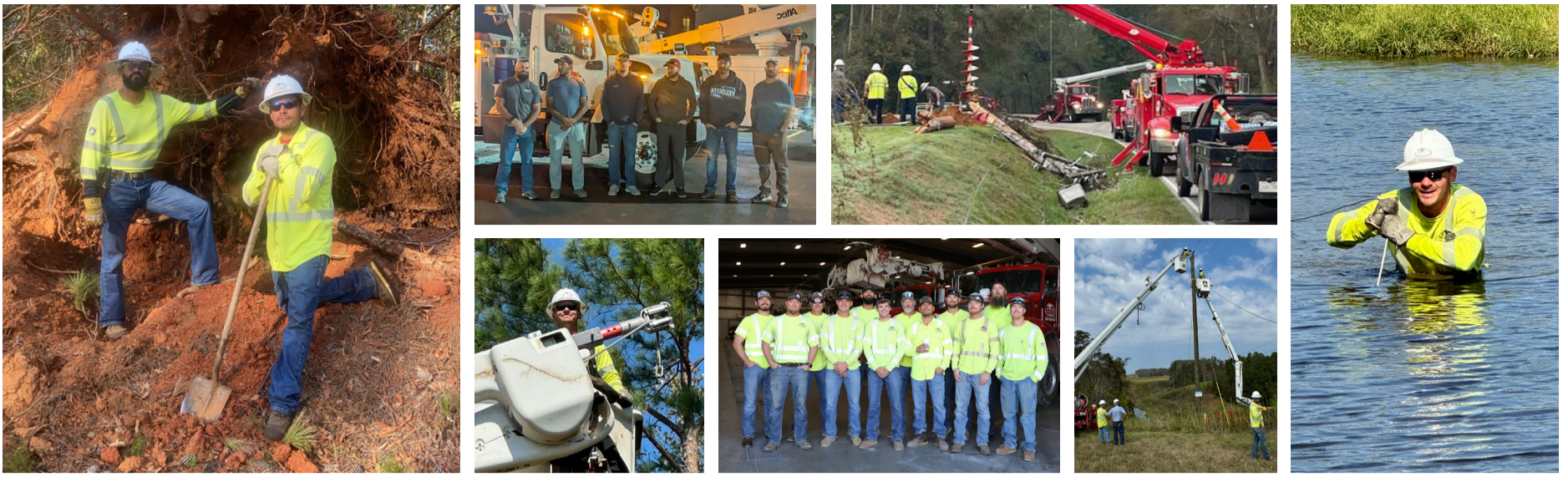
Above: Crews from some of Sunflower's member utilities responded to a mutual aid request from Aiken Electric Cooperative in South Carolina.
